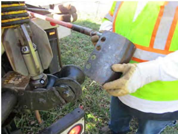
Photo 7-1. Debris Traps and Poles Used to Set Debris Trap in Manhole Channel
