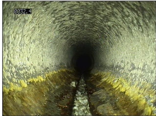
Figure 3. Ductile Iron Pipe Invert Corrosion from Acidic Discharge
