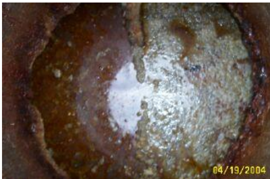
Grease trap baffle wall corrosion
