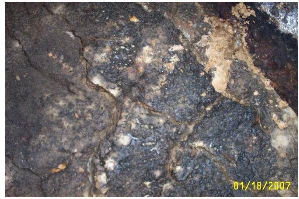
No outlet T located due to depth of FOG, no Grease trap maintenance! Noncompliance
