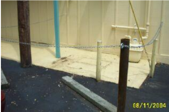
Under vault top, 250 gallon customized GI
