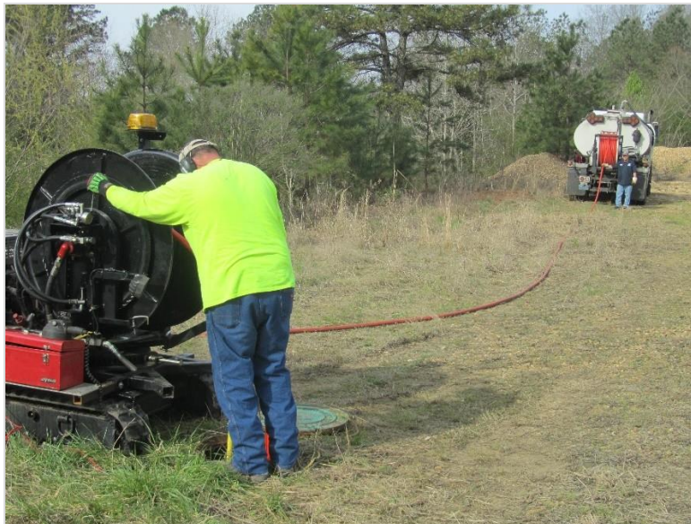
Figure 3. JCESD Jet Wash Truck and Easement Machine
