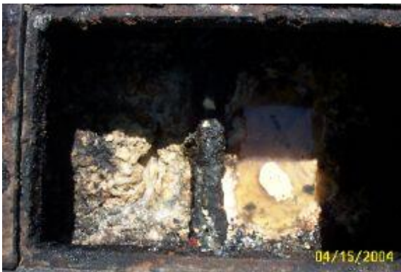
Small 30 gallon outside floor trap w/ heavy FOG, no Ts
