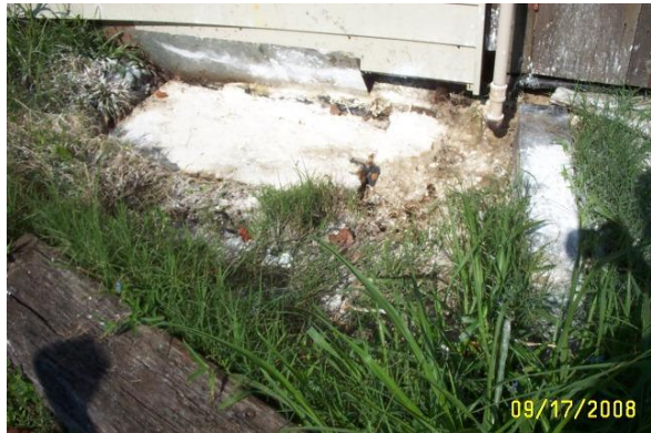
Outside trap with lime covering top due to recent Overflow
