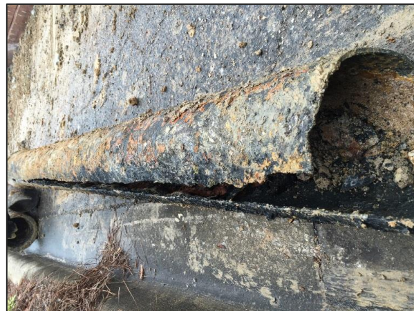
Figure 2. Ductile Iron Pipe H 2 S Corrosion
