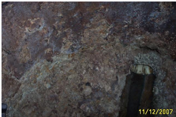
Hydrogen sulfide damage in manhole
