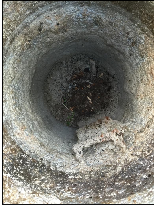
Figure 1. Concrete Manhole Corrosion from H 2 S Gas
