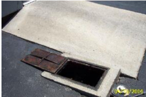
Small 50 gallon outside floor trap
