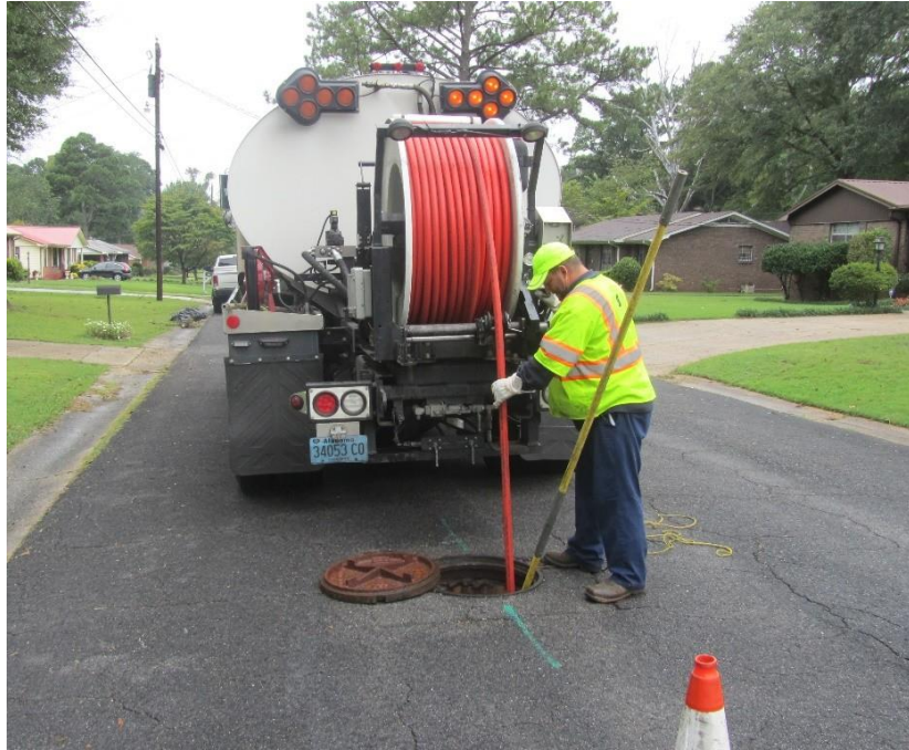
Figure 1. JCESD Jet Wash Truck
