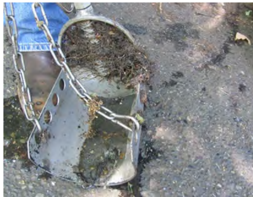
Photo 7-6. Examining a Debris Trap for Signs of Light Roots
