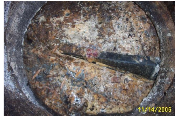
Floating flexible plastic "U shaped" outlet T that has become dislodged from the trap wall.
